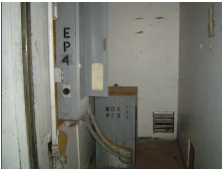
Transformer located in north end of building – labeled “Non PCB.”
