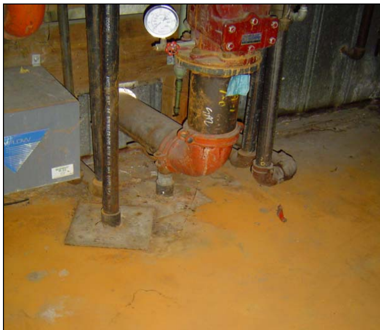
Pump located in building with rust/copper debris surrounding on concrete.
