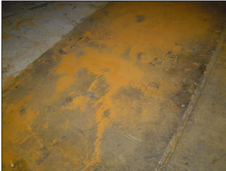
Observed rust or copper debris on concrete in building.
