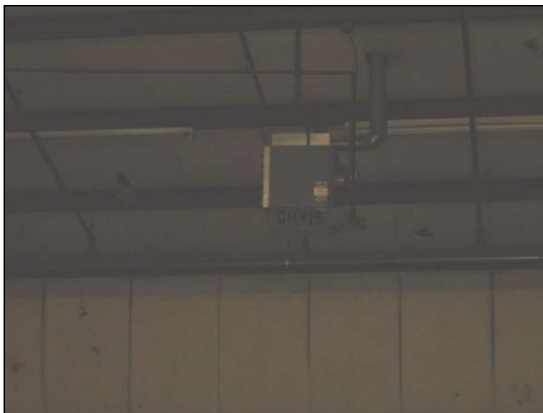
Air circulating device hanging from ceiling in south end of building.
