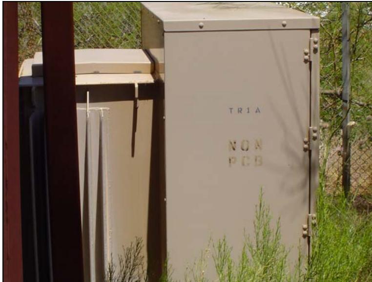
Transformer located outside northeast end of building – labeled “Non PCB.”
