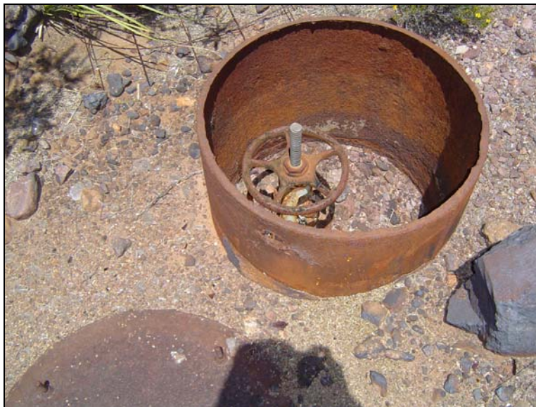
Valve located outside along west side of building.
