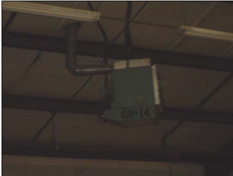
Air circulating device hanging from ceiling in south end of building.
